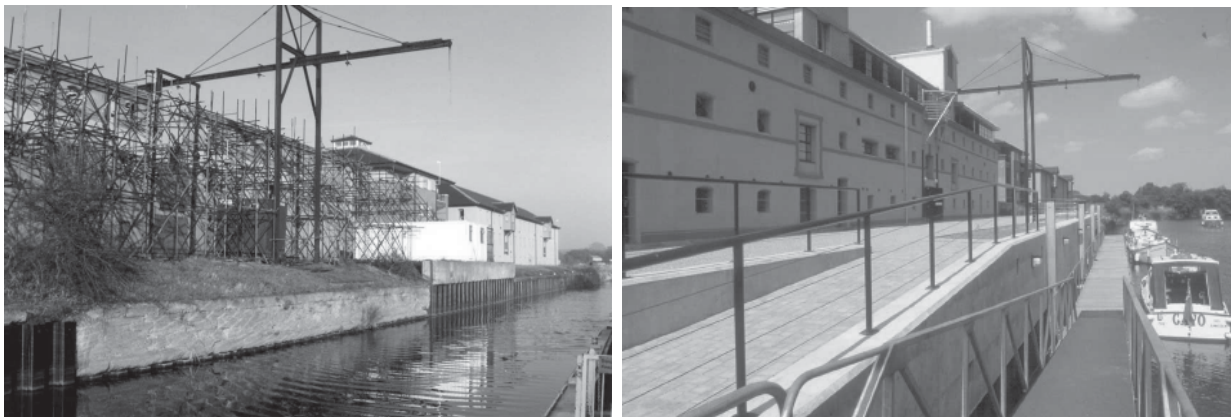
Fig. 4 The Grade II* listed Maltings at Newark Riverside before and after repair and conversion. These are mid 19th century mass concrete buildings, one of the earliest example of this construction type. Fire damaged and long-term BaR they were converted by British Waterways in the late 1990s to become their regional offices. The restoration of these buildings has acted as starting point for further regeneration of the riverside.
